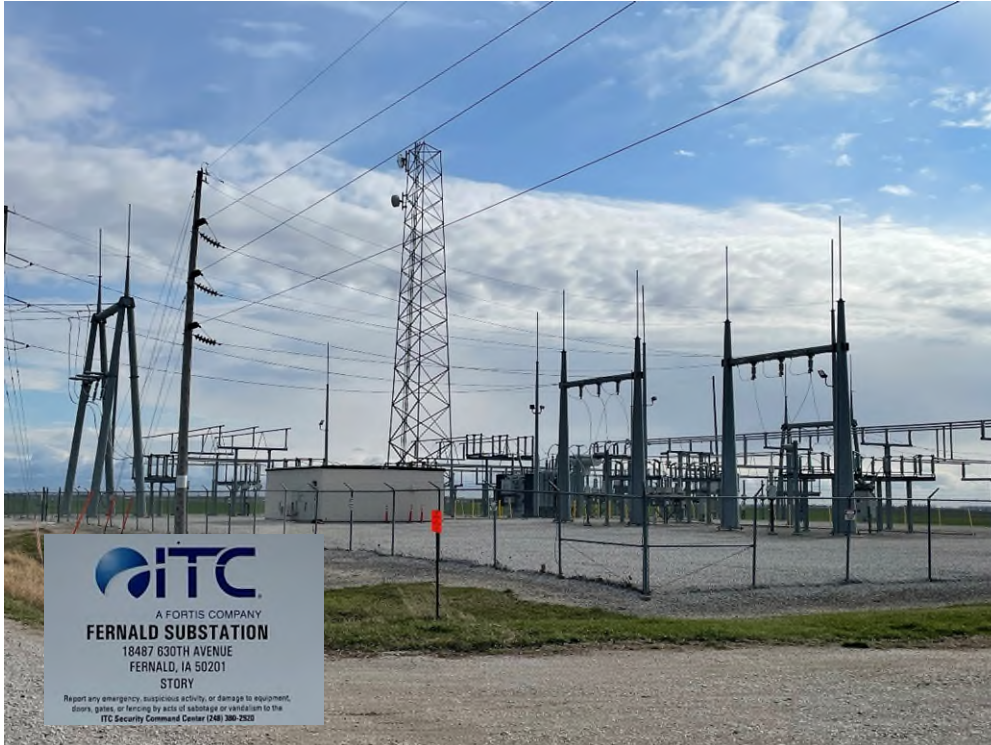
ITC Midwest's Fernald substation northeast of Nevada.
